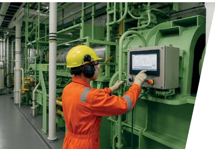
Engine room operations monitoring
